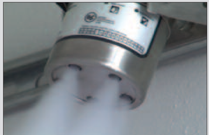
Stat-X® unit discharging.
