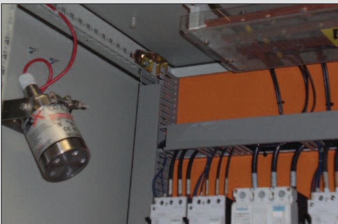
Electrical cabinet protected with a Stat-X® extinguishing system.
